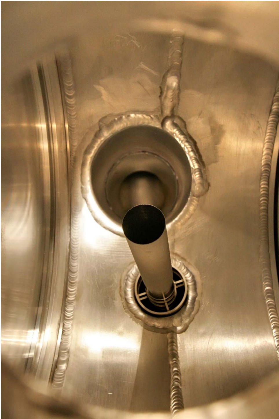
Lens mounted in converter chamber
